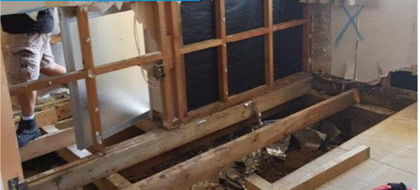
Water damage to the Mangere property
